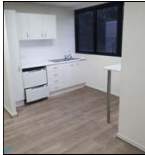
Kitchen area at the back of the building, above left, and toilets, including ambulant toilet, are adjacent to the kitchen.
